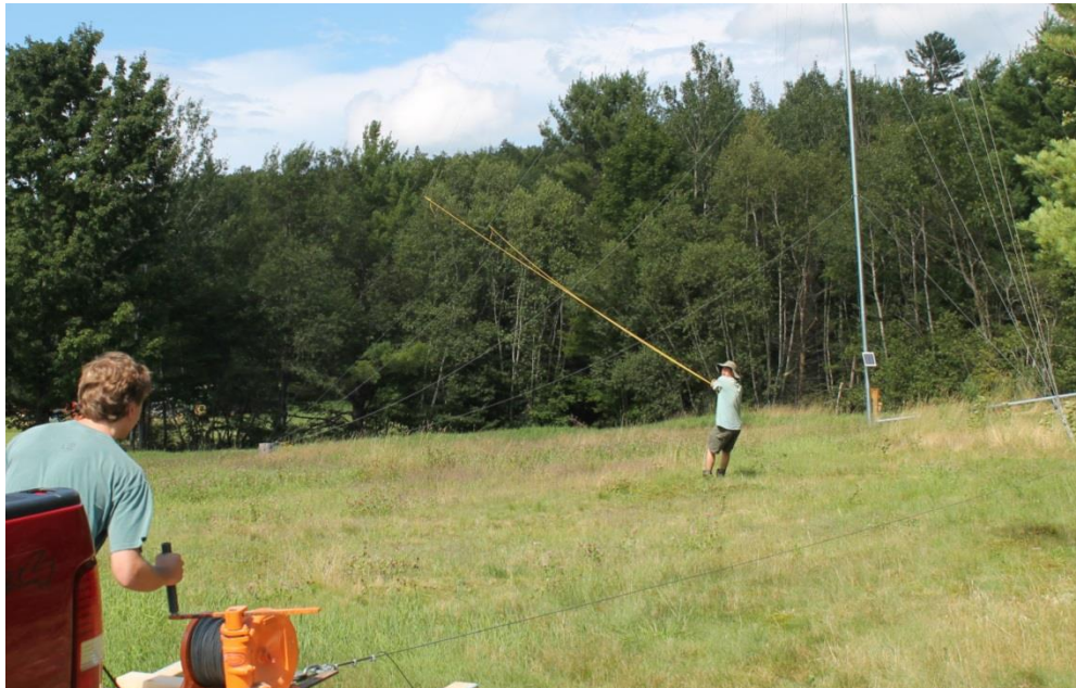
Figure 6.1 – Use of front guy tension ropes during raising of tower to prevent the tower from crashing into and beyond the vertical position. Note heavy duty worm drive winch and redirection of raising cable through use of an optional 5 th anchor at end of gin pole.
